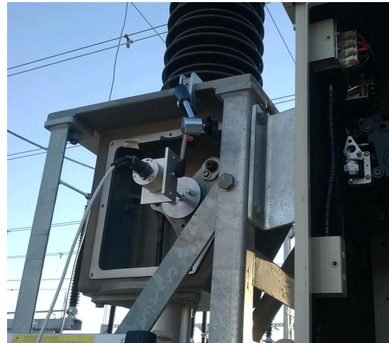
Digital rotary transducer mounted on ABB LTB 245 kV SF6 circuit breaker
